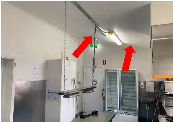
Above: Water damage to the ceiling at the south end of the kitchen.
