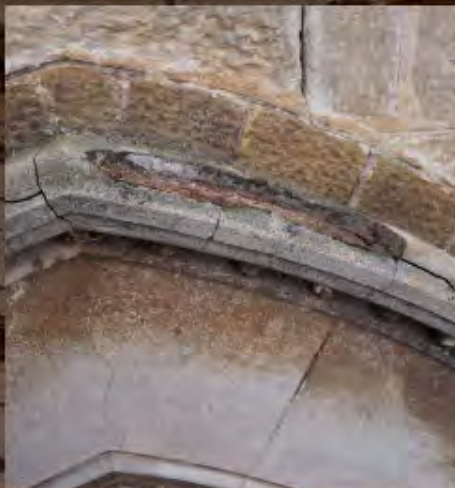
Above: Embedded iron fixing rusting and cracking a surrounding stone moulding that is now in danger of falling from height.
