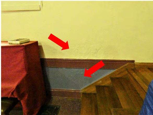
Above: Blistering paint at the base of the wall into the north east corner adjacent to the steps onto the stage.
