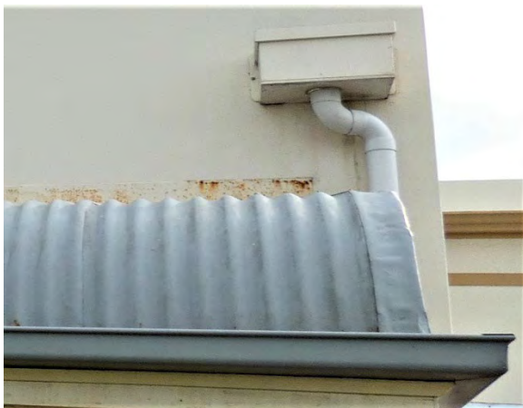
Above: Rusting abutment flashing to the roof of the east verandah. Note the galv rainwater head and uPVC downpipe. The gutter appears to be Colorbond. The gable flashing is painted lead.
