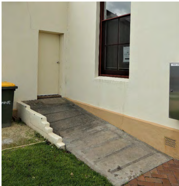
Above: If the ramp to the south kitchen door is redundant it would be best to remove it.
