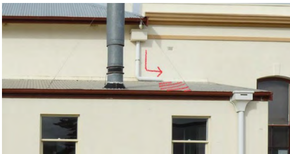
Above: Water draining from the upper roofs is concentrated onto the south end of the kitchen roof. The uPVC drainage pipe does not appear to be a spreader.
