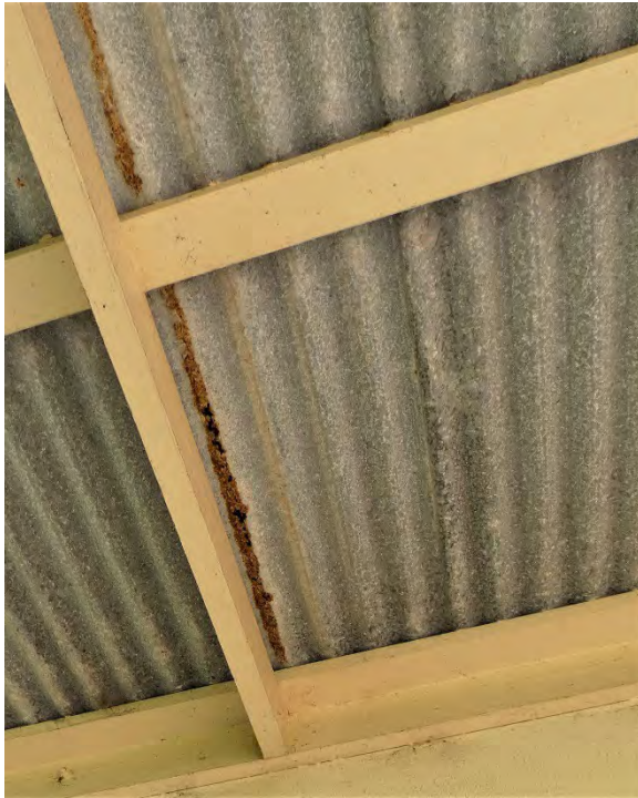
Above: Rust at junctions between galv roof sheets seen only be seen on underside of the east verandah.
