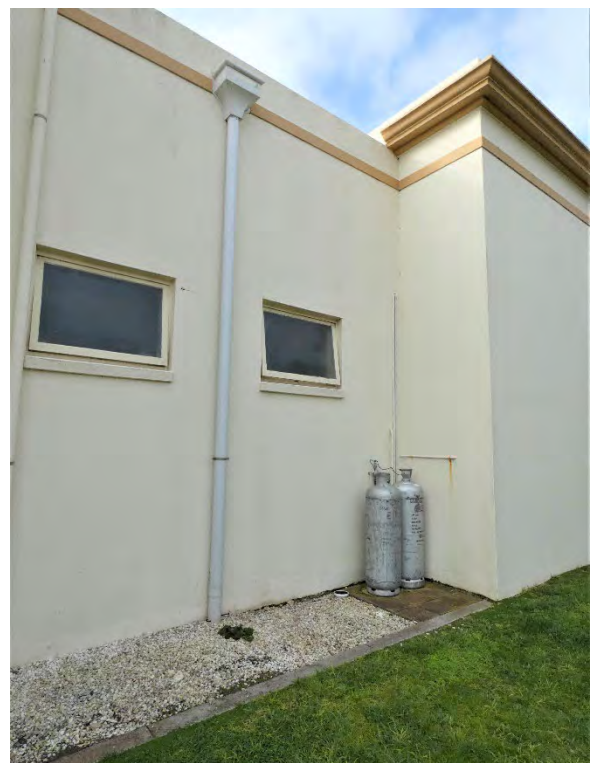
Above: Gas bottles on the south elevation.
