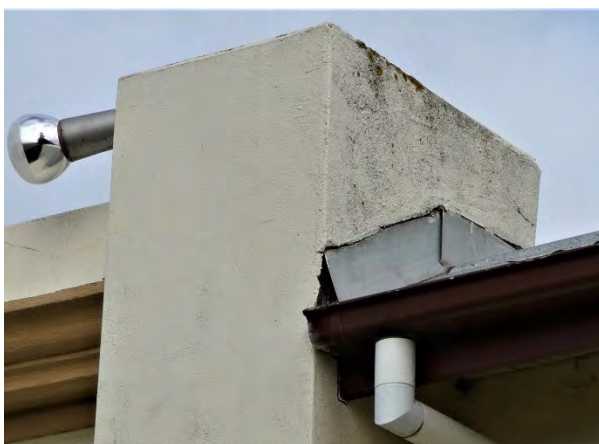
Above: Poor abutment flashing detail at the east end of the hall roof where it meets the library roof along the north elevation. The flashing is not properly sealed against the wall.
