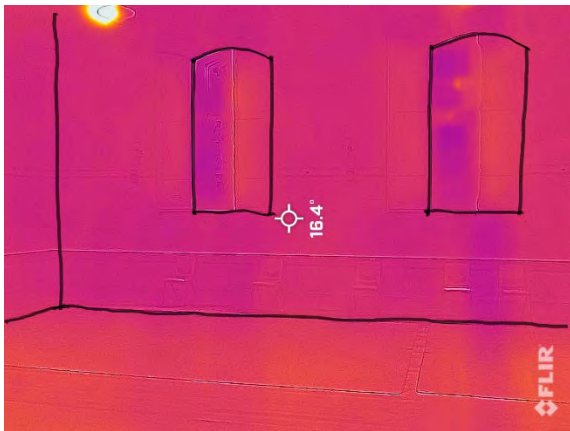
Above: Thermal image looking into the north west corner of the hall. The purple, as opposed to red/ orange colour, indicates a lower temperature where moisture evaporating from the wall surface cools the wall slightly. The window glazing can be seen as purple also.
