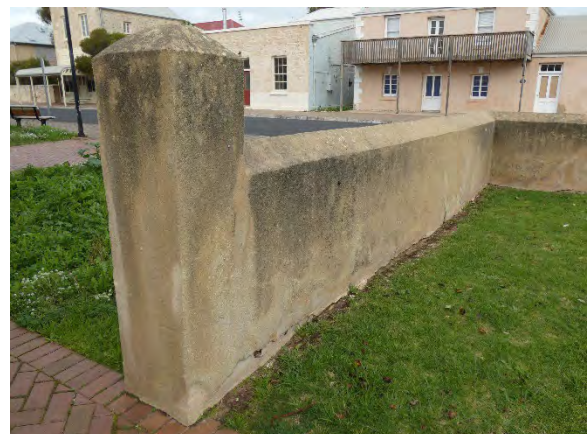
Above: The cement render to southern walls requires repairs.
