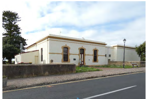
Above: The uniform render and paint does not delineate the newer extensions from the original Institute building.
