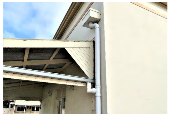
Above: Missing area of diagonal boarding on the gable of the east verandah roof.
