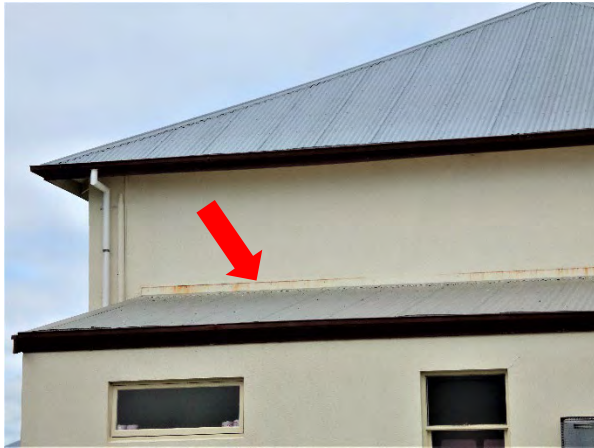
Above: View of north west corner showing D-profile painted galv eaves gutters. Note the rusting abutment flashings to the lower roof.
