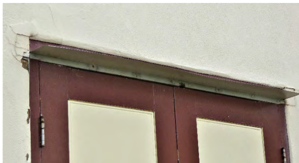
Above: The render is failing at both ends of the lintel to the northern door into the hall.
