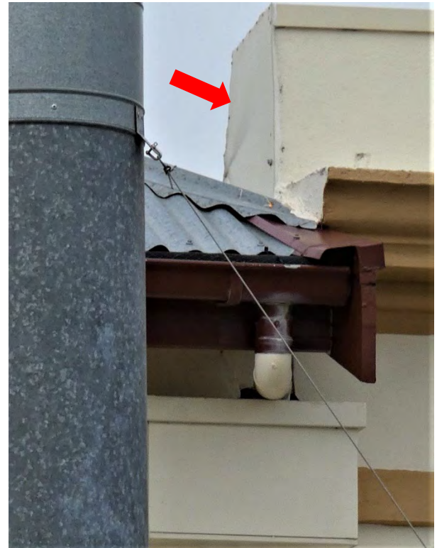
Above: Poor abutment flashing detail where a Colorbond flashing has been rivetted and screw-fixed to the end of the upper parapet wall.
