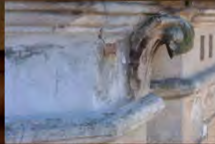
Above: Decorative stonework on an Adelaide heritage building. Note the exposed and rusted iron fixing with a surrounding cement repair. This is where stone features have formally been located and have either been removed for safety reasons or have fallen off.
