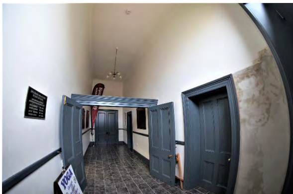
Above: Entrance lobby looking from the front door. The recent plaster repair can be seen on the right side of the image.
