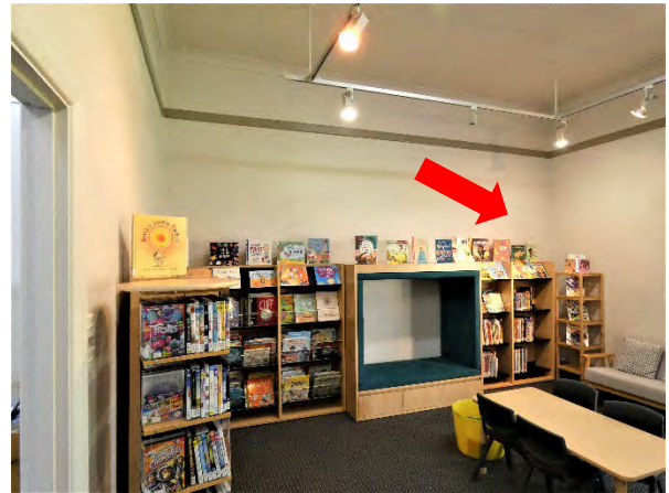
Above: Red arrow indicates where the paint is blistering from moisture drying out through the wall surface.
