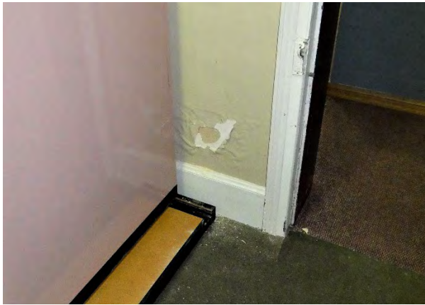
Above: Blistering paint at the base of the wall behind the compactus.
