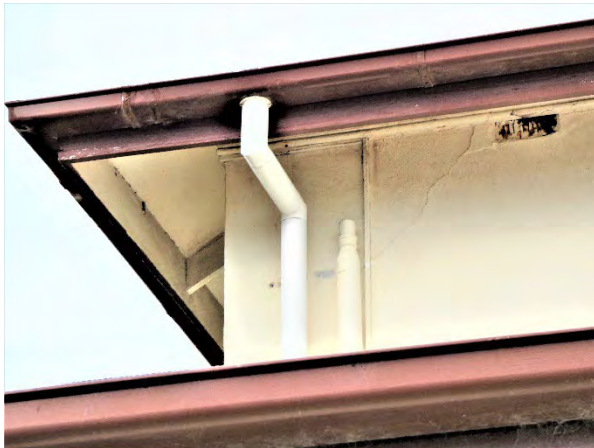
Above: A closer view of north west corner showing that the galv gutter and brackets to the top hall roof are badly rusted.
