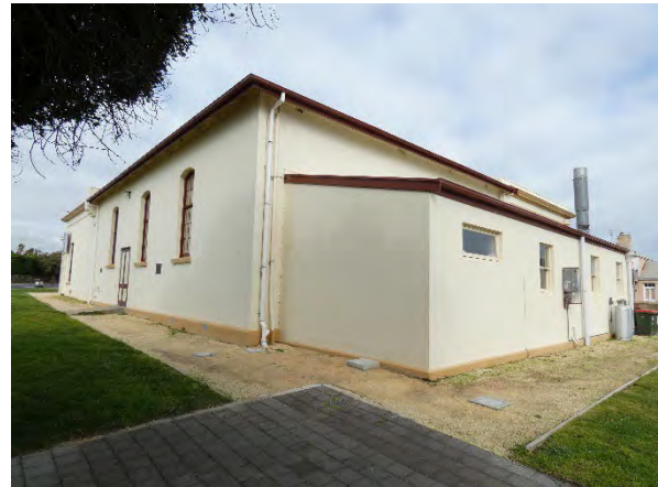
Above: Damp gravel strip along north, west and east elevations.
