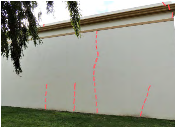
Above: East end of south elevation indicating the most obvious cracks the in render.
