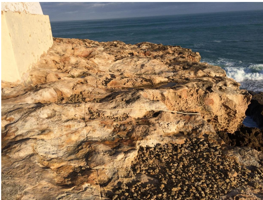
Photo 6: View looking west at the northern boundary to the Obelisk, noting uneven ground and a long crack between the Obelisk and the white 2m length tape.
