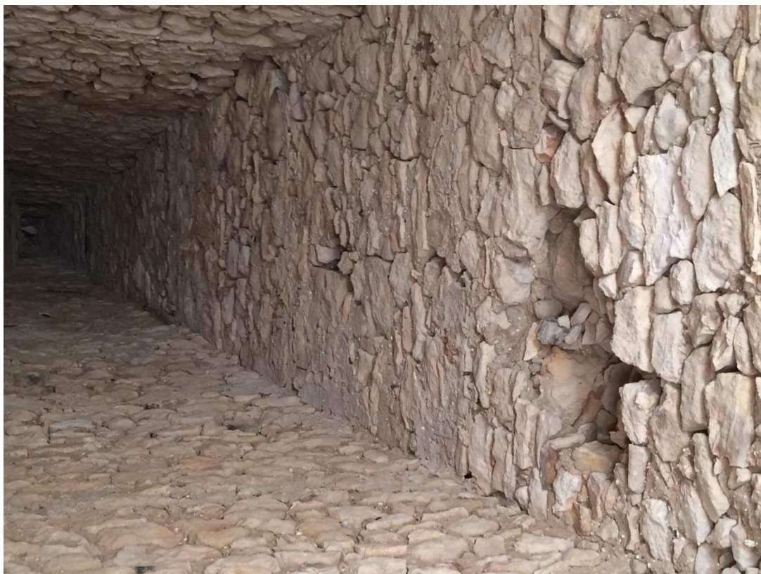
Photo 5: photograph of internal northern wall where a segment (approx. 1\text{m}^2 ) has a significant weakening. Location is approximately at the location of the 1st Red line on the outside of the Obelisk.
